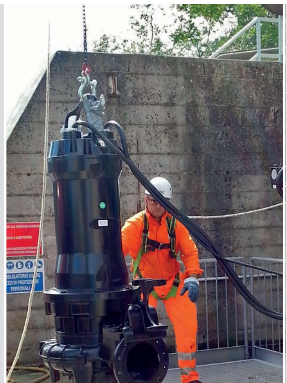
Pumping station for heavily soiled sewage (Italy) Four ZUG CP 250B 45/6 AW pumps
